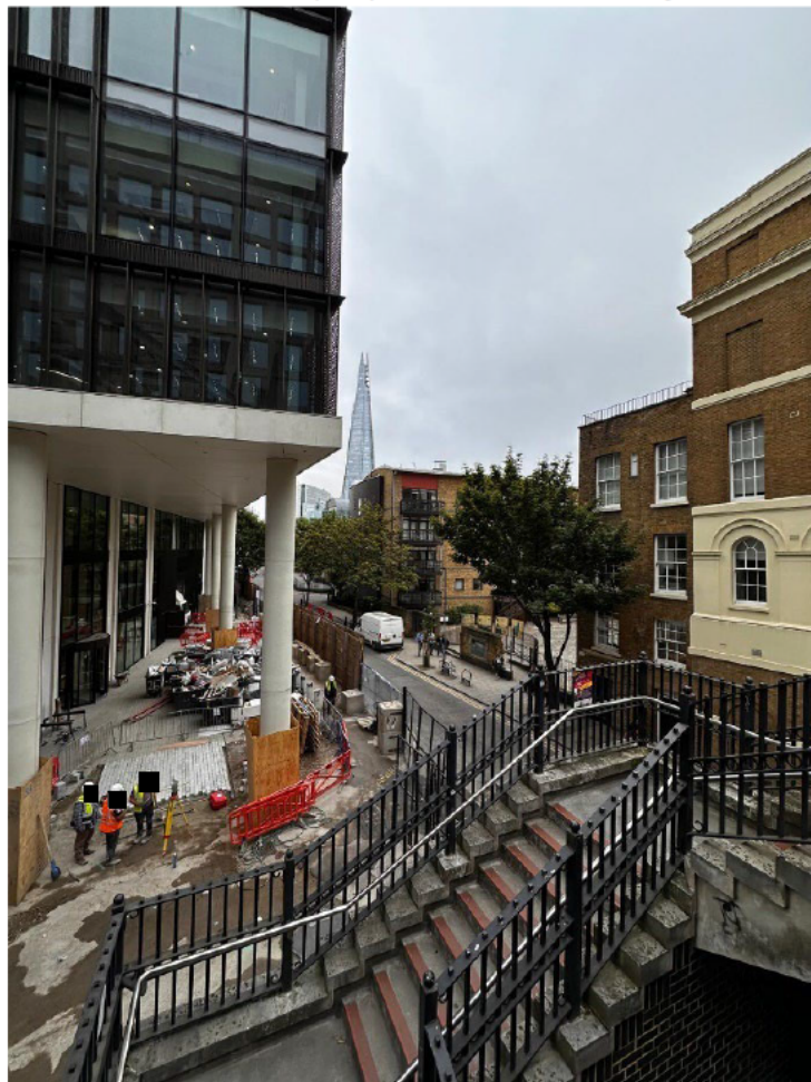
Below is the view of the residences at Old Theatre Court (left) and Anchor Terrace (right) viewed from the proposed terraces, across the narrow road. There is no noise containment between the Level 0 and Level 7 terraces. Without conditions to prevent it, smokers would be likely to congregate here, under residential buildings.
